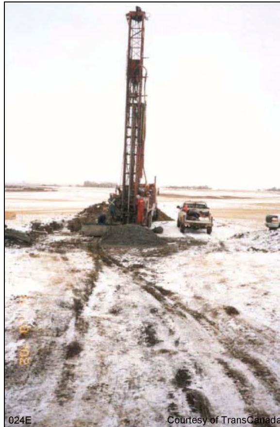
Figure 3-18: Example of a Deep Well Anode Drill
