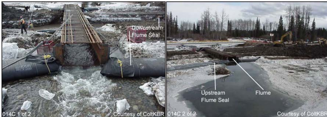
Figure 3-41: Examples of an Isolated Dam and Flume Crossing Horizontal Directionally Drilled Crossings
